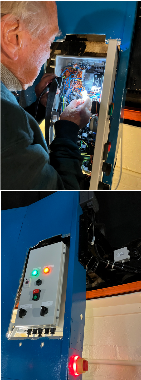
Figure 6 New 12" dome control. (Top:) Alan Bagnall putting the finishing touches; (Bottom:) the final product with the black mains socket at the top right.
